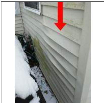
Appears to be melted from Grill
