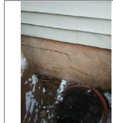
Step crack southwest corner
