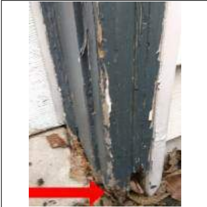
Brick molding garage door damaged
