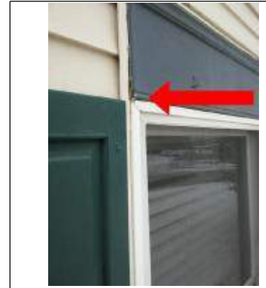
Missing damage caulk
