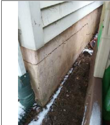
Horizontal step crack southwest corner
