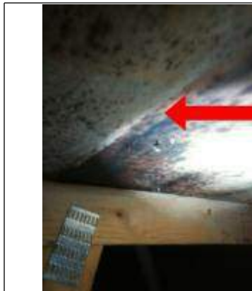
Decking overlapped due to lack of expansion clips
