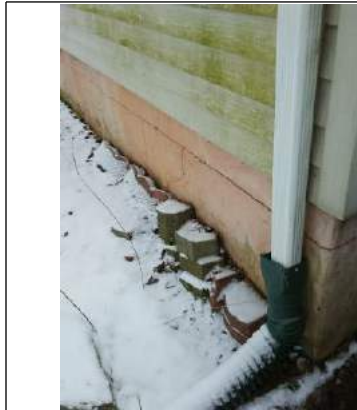
Horizontal crack West
