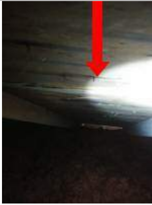
Several areas of roof decking bound up and overlapping
