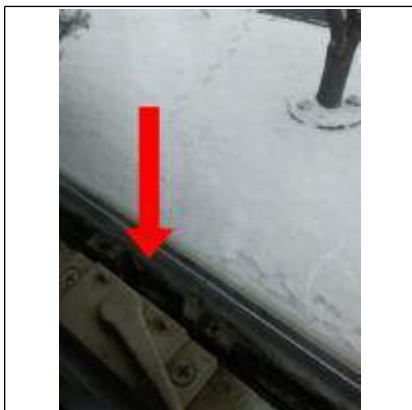
Broken lock mechanism
