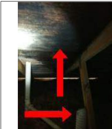
Interior west side of Home mold like substance on roof decking also vent duct work not extended to the soffit causing condensation to fall on interior insulation
