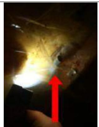
Cut exposed wiring in closet at basement behind family room recommend further evaluation and repair
