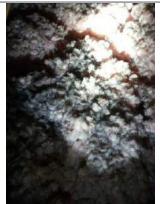
Insulation wet due to condensation falling from interior of decking down source vent not exhausted properly
