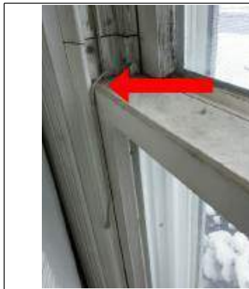
Window balance broken living room right
