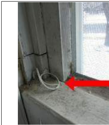
Window balance broken will not stay up living room left
