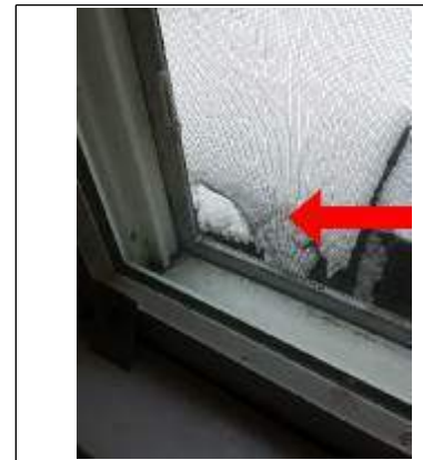
Kitchen window screen torn
