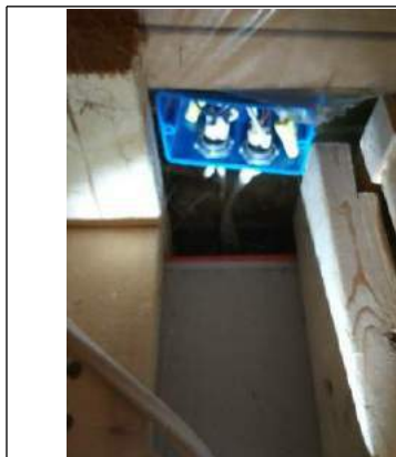
Open junction box in closet behind family room recommend repair see attached photo
